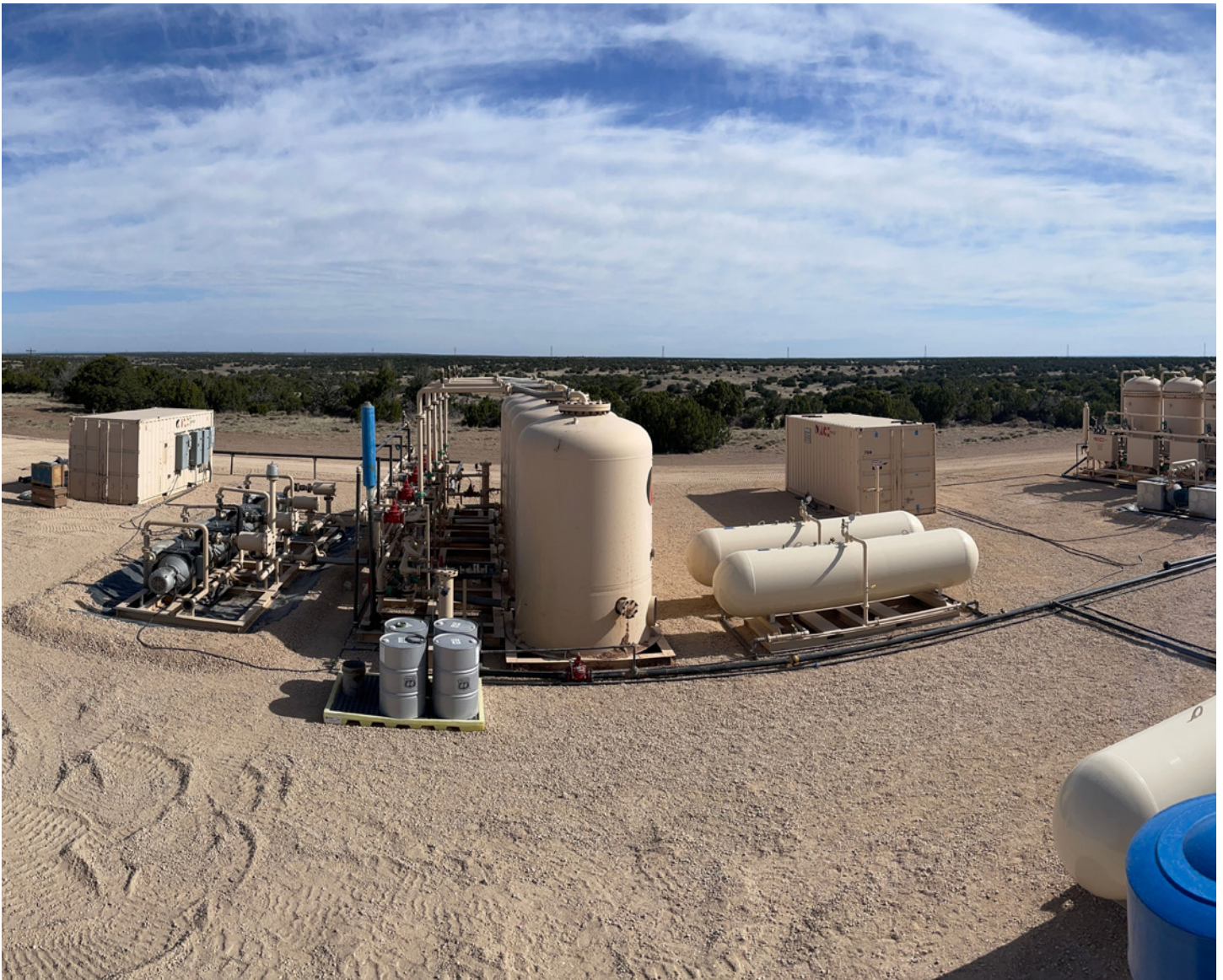
Helium extraction facility in Arizona provided by IACX.
